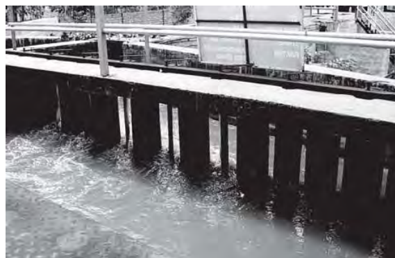
Fig.18.4 Grit and sand removal tank
